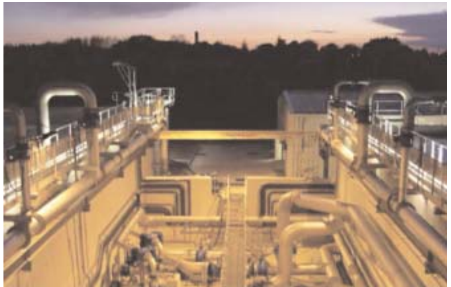
Wastewater Treatment Facility, Bury, Greater Manchester, United Utilities/MHW
