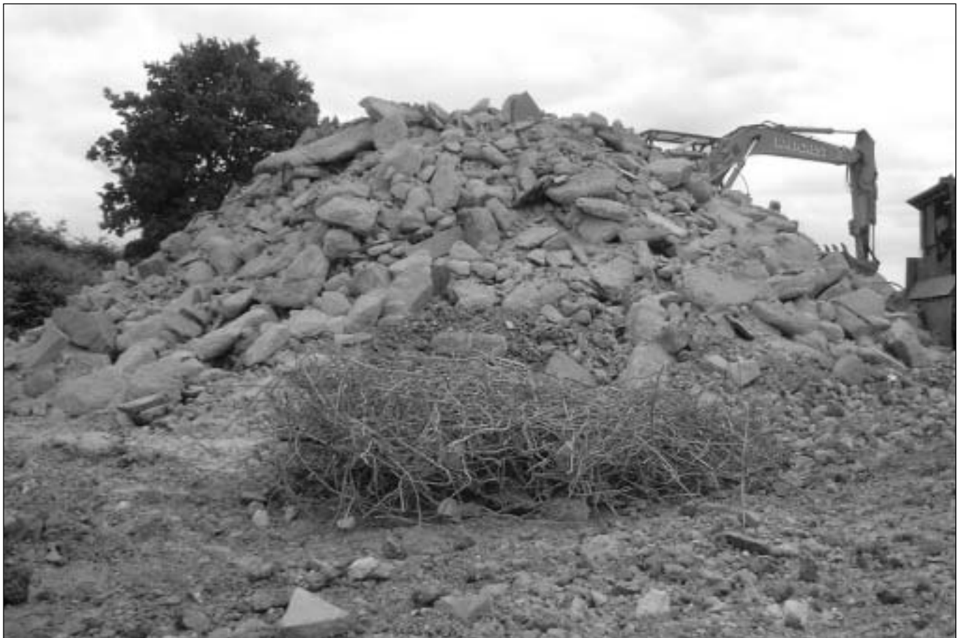
Crushed concrete and segregated steel is recycled for new steel reinforcement and concrete construction.
