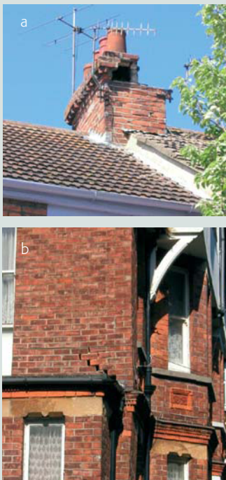
Damage from the 2007 Folkestone earthquake: (a) Damage to a chimney and (b) structural damage, to Victorian masonry houses in Folkestone.
