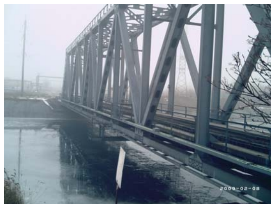
Fig 4 Radioactive railway bridge with a minimum speed limit of 20kph
