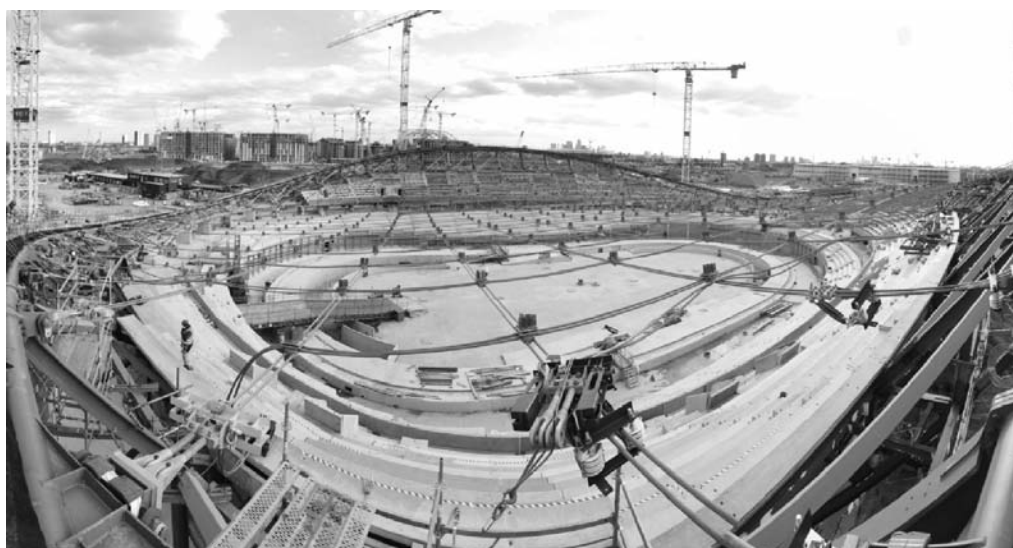
Cablenet roof design at the Velodrome
