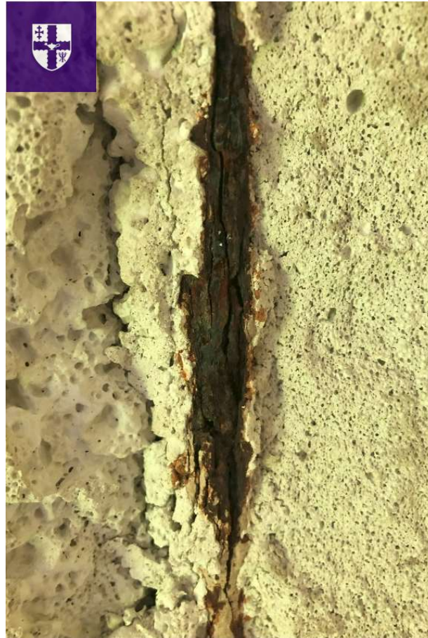
Corrosion in RAAC
