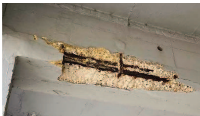
Cracking and spalling due to corrosion of the reinforcement (CPT)
